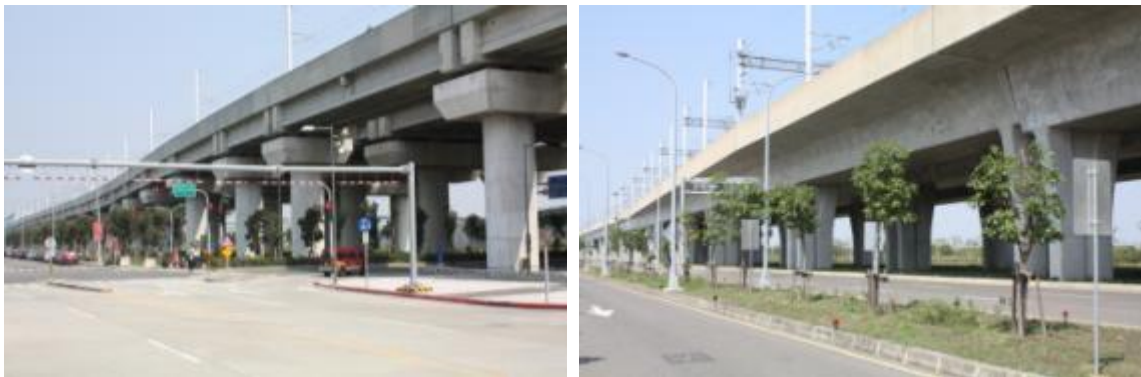
Taiwan HSR: Aerial Structure Variability (note varied columns, caps, girders, sound walls, etc)
