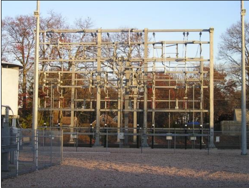
Figure 2-13 Traction Power Substation Overhead Contact System Gantry
