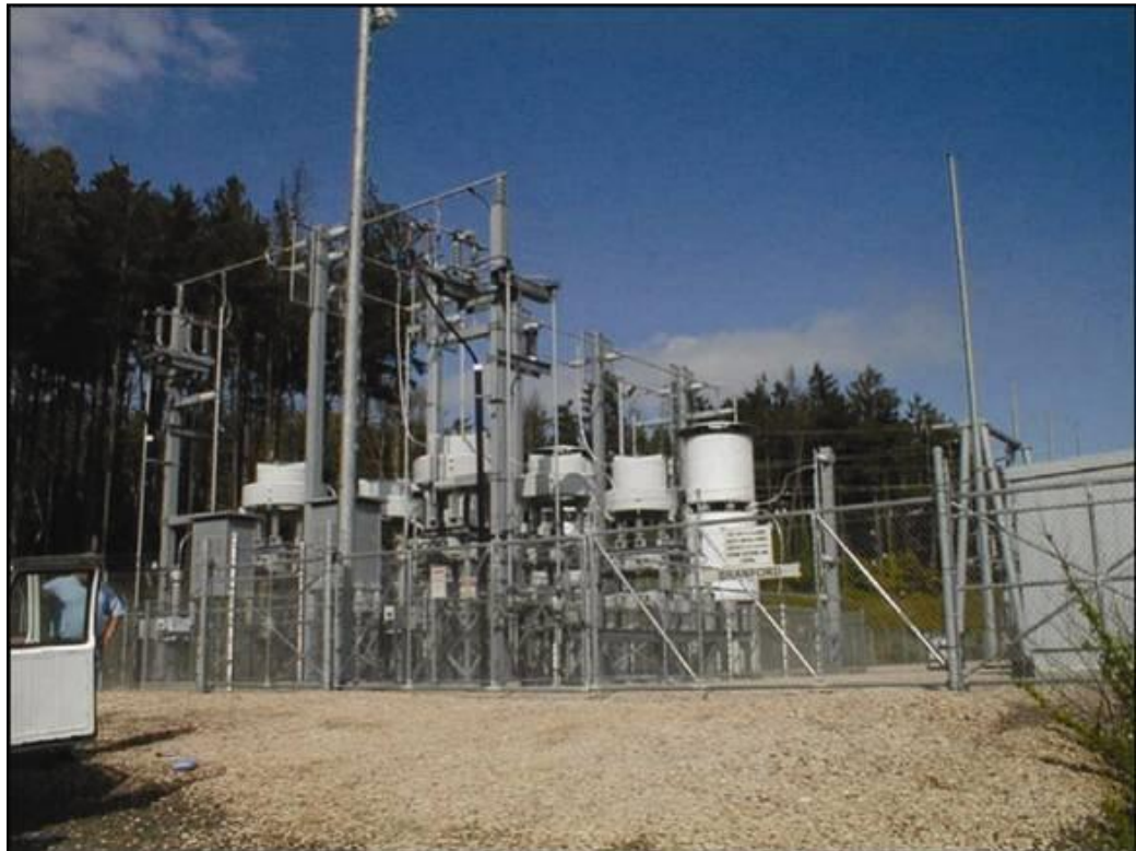
Figure 2-12 Traction Power Substation
