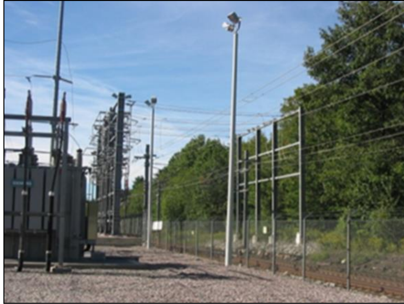
Figure 2-16 Paralleling Station Overhead Contact System Gantry
