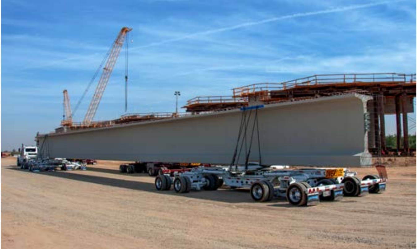
PHOTO: THE ROAD 27 OVERCROSSING WILL BE OVER 700 FEET LONG WITH THE LONGEST SPAN STRETCHING 198 FEET.
