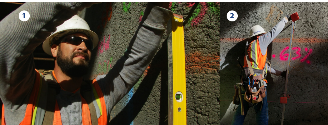
1. Journeyman carpenter Daniel Vara says wet weather didn't stop crews from working on the Fresno Trench, a one-mile underground passage that will carry high-speed rail under State Route 180 near downtown Fresno.
