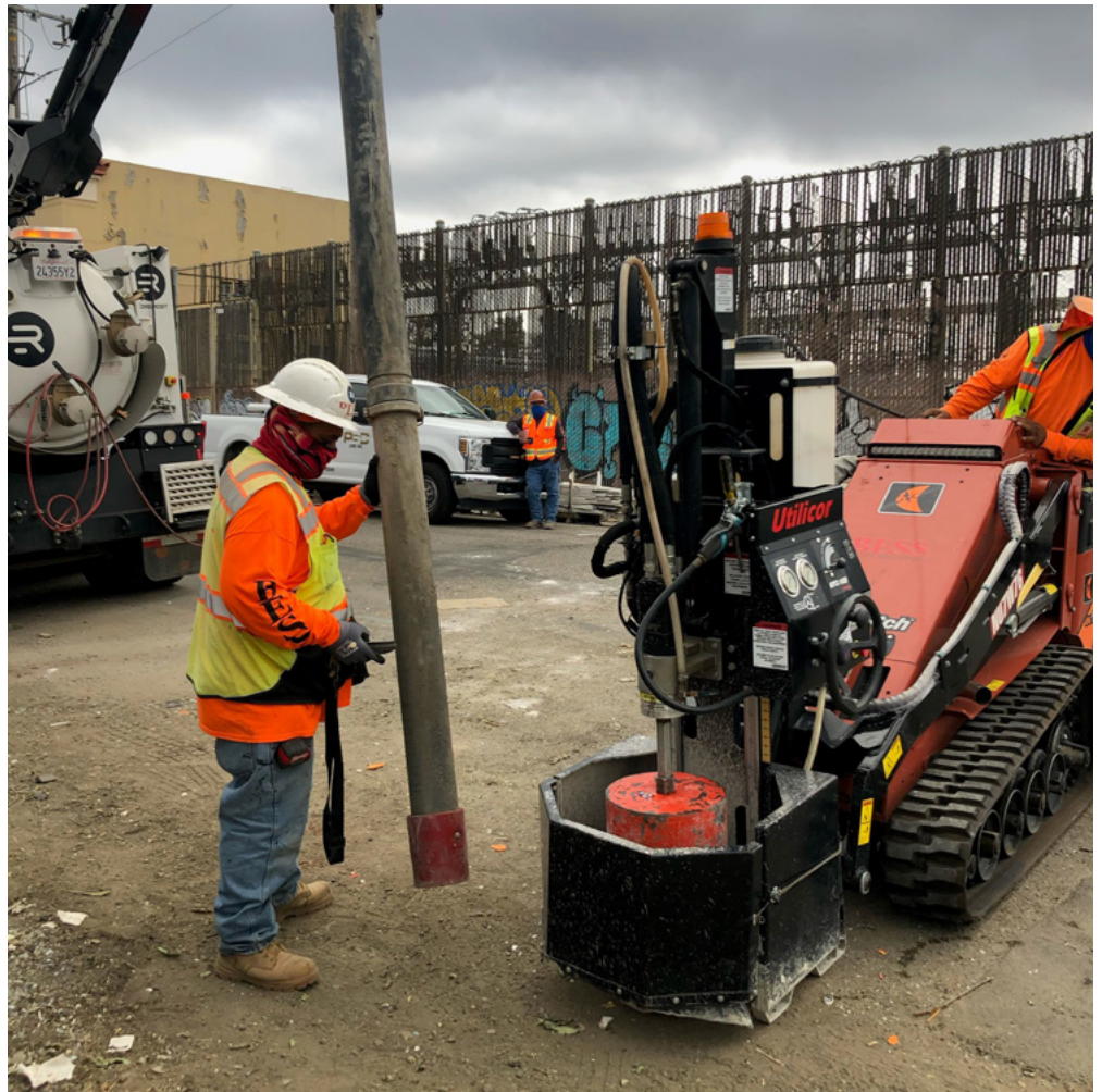
A Bess Utility Solutions crew prepares to drill a hole in the ground using Keyhole technology. The equipment can safely and accurately bore through asphalt and concrete surfaces. The company has been locating, mapping and moving underground utilities for more than 25 years.
