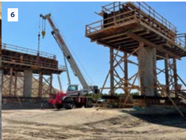
5. & 6. At Fargo Avenue in Kings County, crews worked on bent caps that sit on top of columns for the future grade separation. Eventually, it will take traffic over high-speed rail lines east of State Route 43 and north of the city of Hanford.
