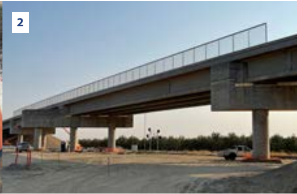
1. & 2. Workers have completed the Road 27 overcrossing in Madera County. Located between Avenue 17 and Club Drive just north of Madera, it's one of nine grade separations in Madera County. It will take traffic over the existing BNSF rail line and future high-speed rail trains.
