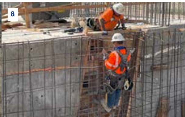
7. & 8. Working on the Peach Avenue structure meant late nights for construction crews. It took them 14 hours to place more than 720 cubic yards of concrete and form the deck. After that, workers sandblasted steel rebar to prepare for the installation of parapet walls.
