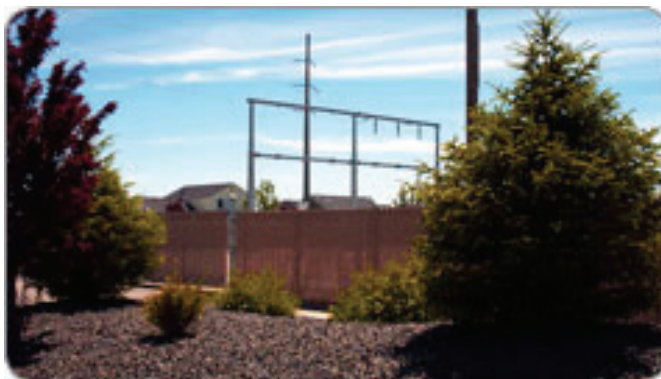
Figure 3.16-29 Example of Power Substation in Urban Setting, with Landscape Screening and Fence
