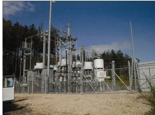
Figure 2-15 Traction Power Substation
