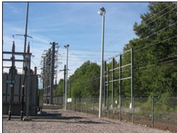
Figure 2-29 Paralleling Station Overhead Catenary System Gantries
