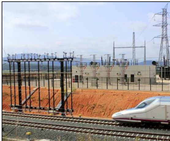
Figure 2-25 Traction Power Substation
