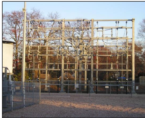
Figure 2-26 Traction Power Substation Overhead Catenary System Gantry
