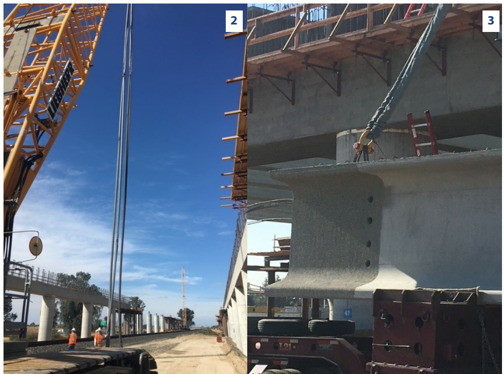
2. Contec Hoist and Rigging provided the lifting slings needed to place girders at the San Joaquin River Viaduct and Pergola.
