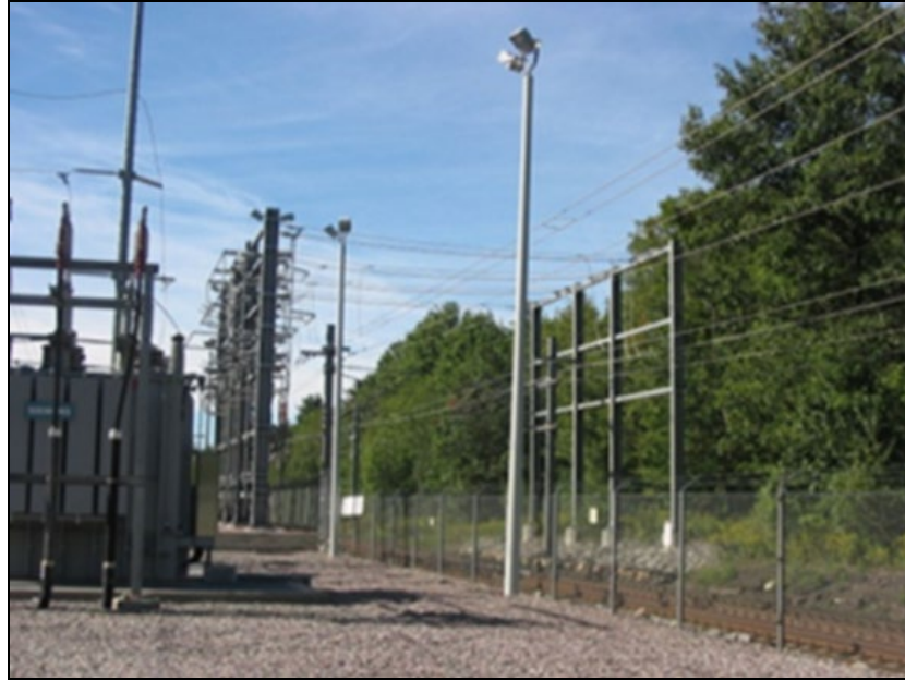
Figure 2-16 Paralleling Station Overhead Contact System Gantry
