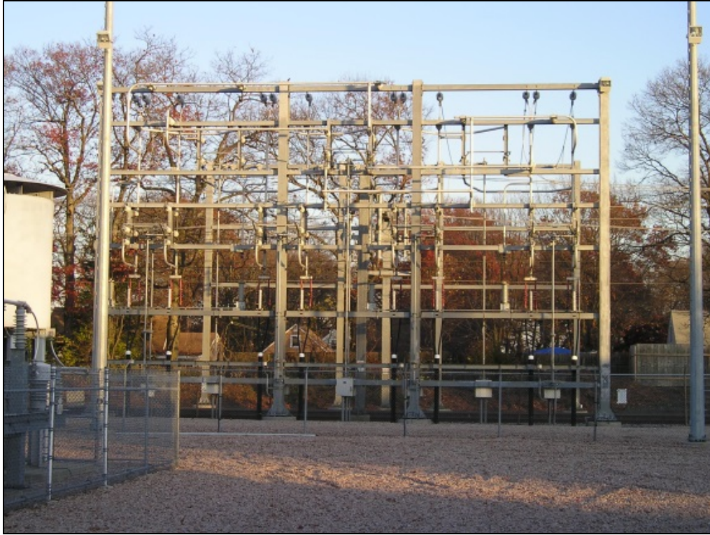
Figure 2-13 Traction Power Substation Overhead Contact System Gantry
