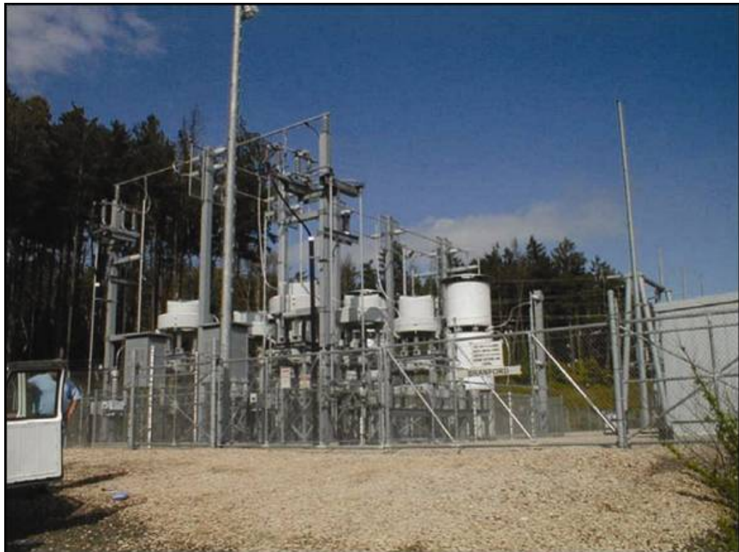
Figure 2-12 Traction Power Substation
