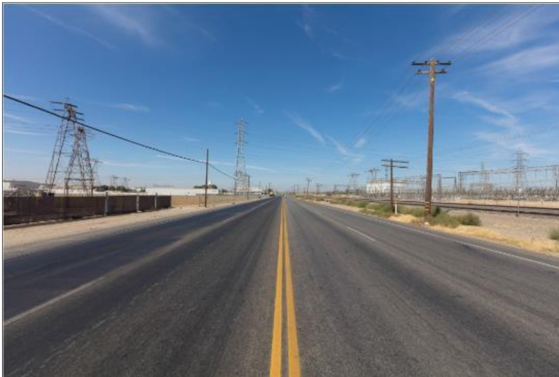
Figure 4-5 Magunden Substation Vicinity, Existing Site—Camera Facing West. The VERs would relocate the existing towers at left further south to make space for a traction power station.
