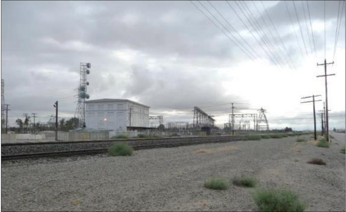
Figure 4-3 Magunden Substation and Vincent, Big Creek East, and Big Creek West Transmission Lines, East Bakersfield
